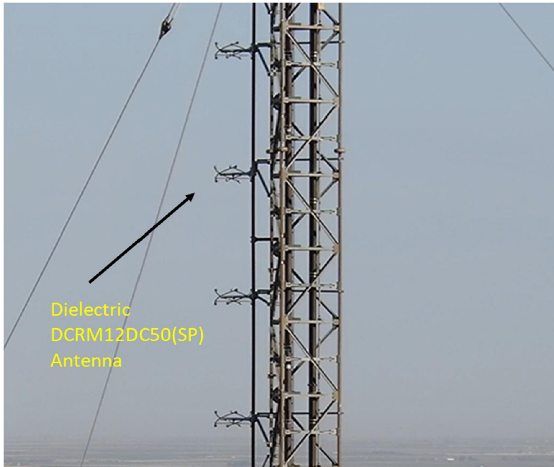
FIGURE 4: DCRM12DC50(SP) ANTENNA INSTALLED FOR KLBB-FM, KTTU-FM AND KXTQ-FM IN LUBBOCK, TEXAS.
