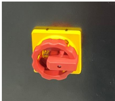
Figure 1: Main shut off switch with Lock Out Tag Out (LOTO)
